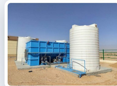
■ Packaged treatment units and pumping manifolds across the corridor.
