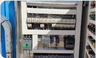
Motor-control-center assembly under workshop conditions — structured wiring, labelled terminations and protection settings verified before site energization.
