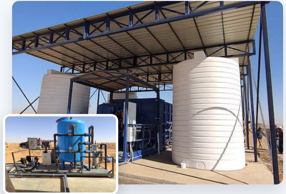
Packaged treatment train and station works under utility supervision, Toshka corridor.
